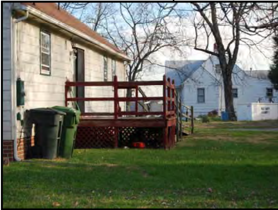
Deteriorated Rear Deck on Corner Lot
