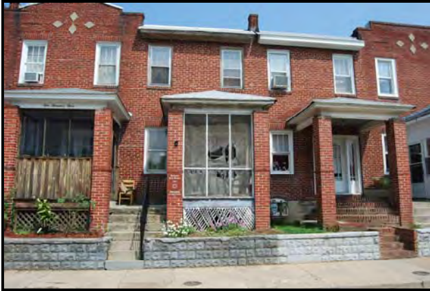
Deteriorated Porch (center home)
