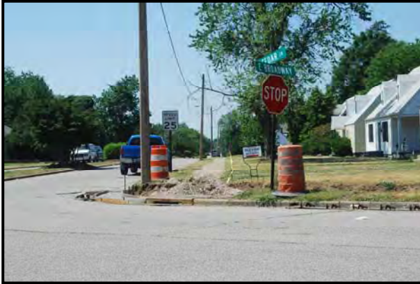
Lack of curb cut- inaccessible to handicap
