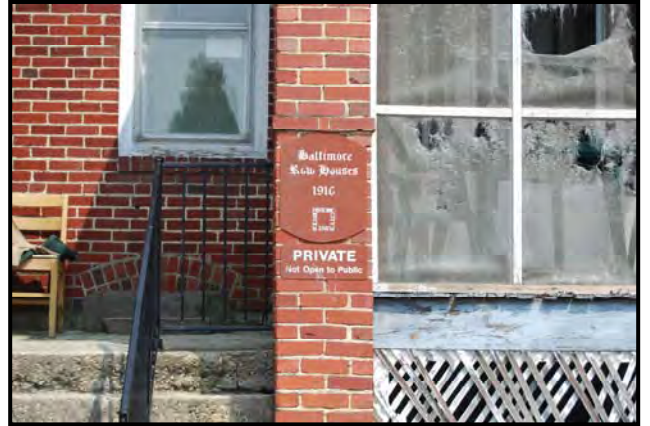
Deteriorated Porch flooring/cement steps
