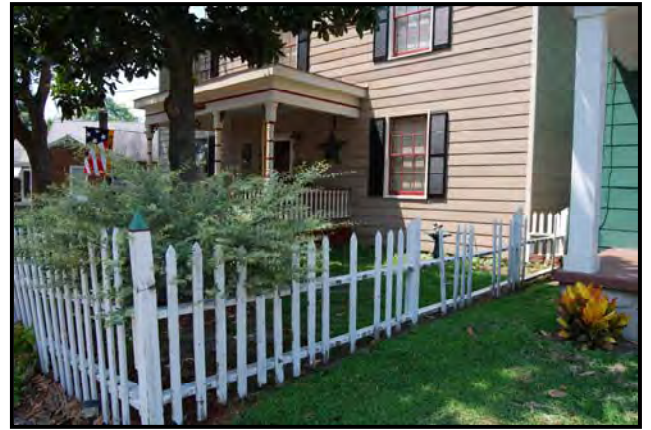
Deteriorated fence from the east of home
