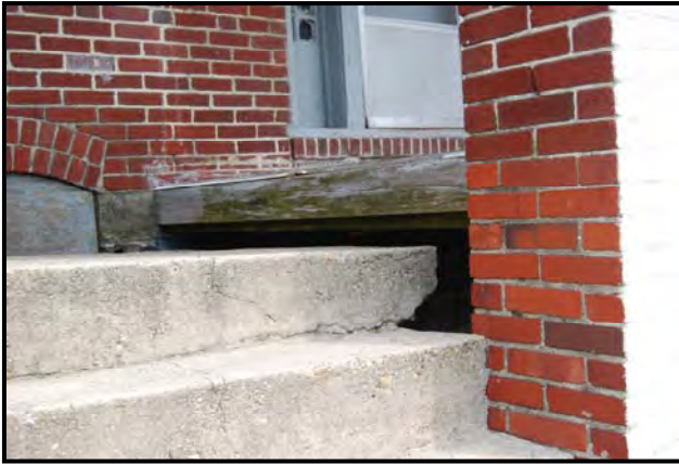
Steps separated from porch and home
